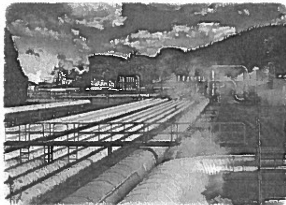
Geothermal power station.
